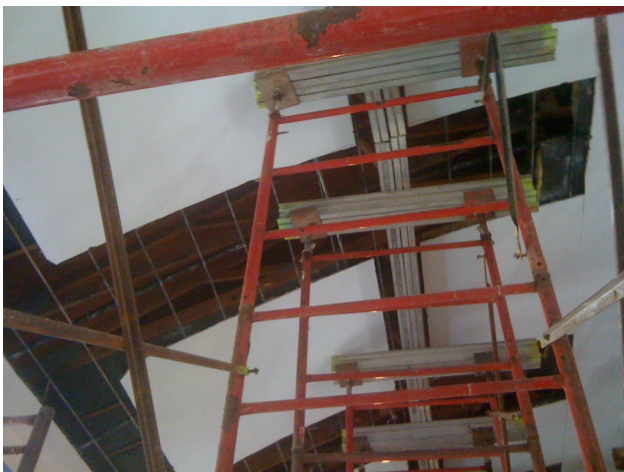
A cross seemed to form from the ceiling reinforcement.
