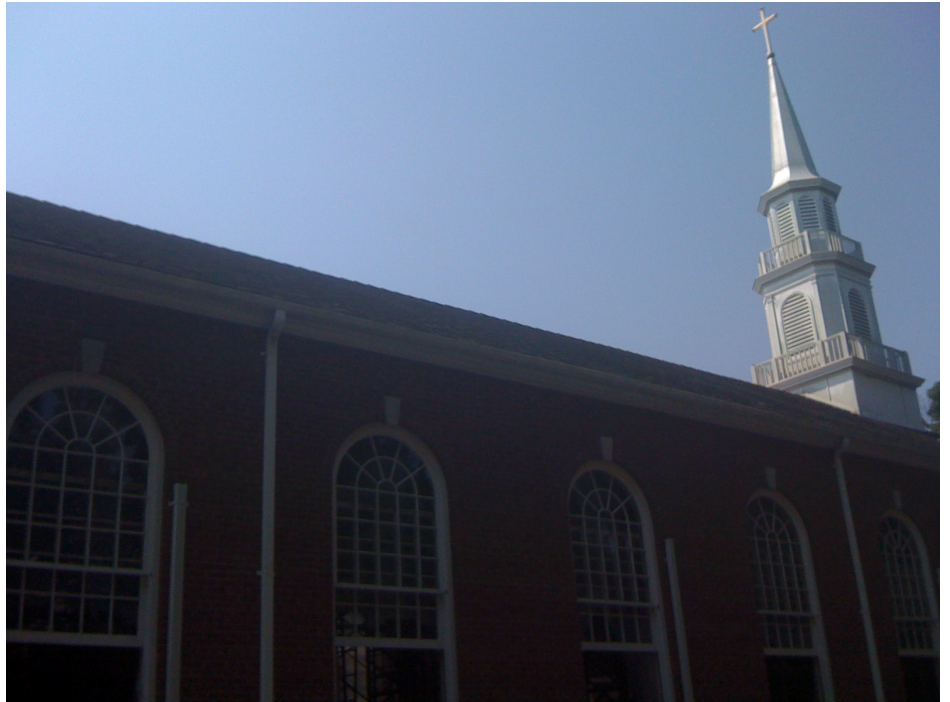
The roof ridgeline is straight and the walls are back in position.
