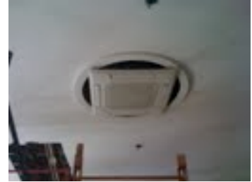
New HVAC Unit in Loft
